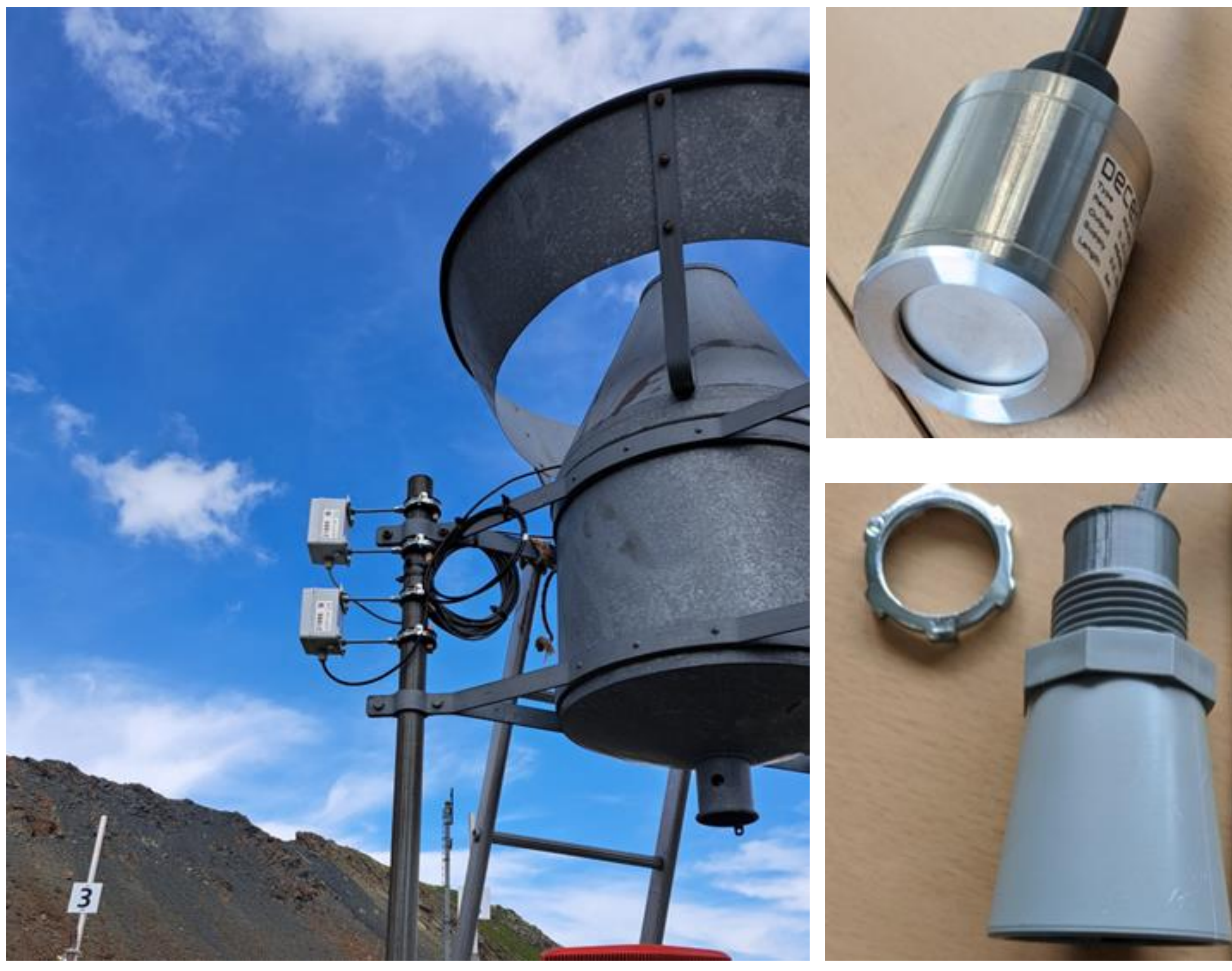
Fig. 2: The boxes containing the electronics for the pressure (right above) and the ultrasonic sensor (right below) were attached to a support of the totalizer (left), pointing towards the LoRaWAN antenna.
